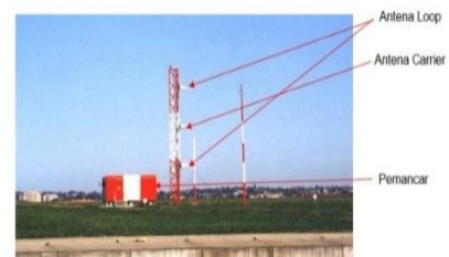
Gambar ground antenna glide slope
